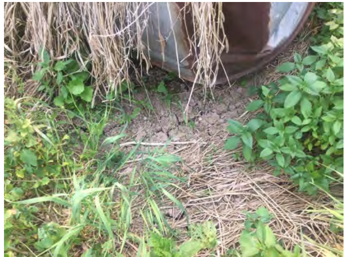
mud cracks near culvert, change in vegetation.
